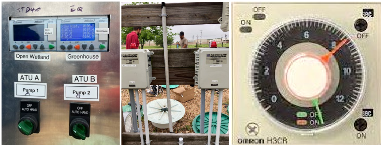
Figure 18. Direction of flow from the trash tank to the two ATUs and two drip lines being compared (top), meters monitoring the flow to the ATUs (bottom left), and control panels and Omron timer controlling the flow from the aeration tanks to the pump tanks (bottom right).
