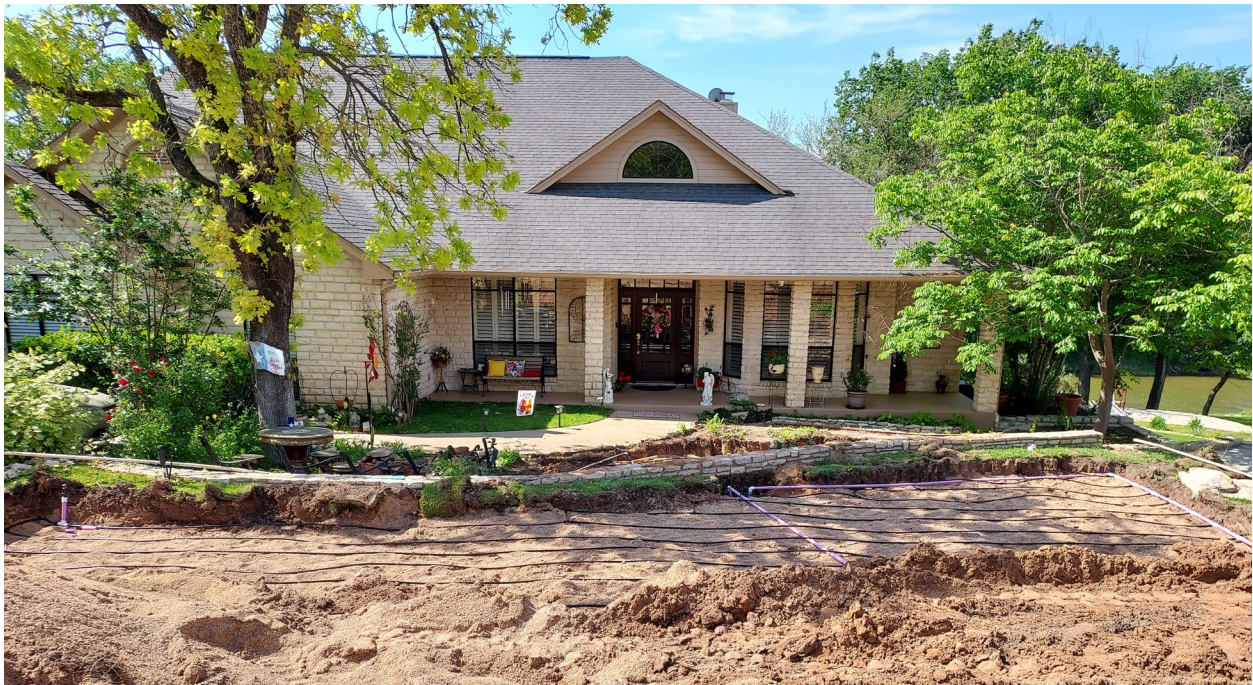
Figure 12. New way of doing it – Using gravel as bedding materials. (Site # 1-2). (Photo Anish Jantrania).
