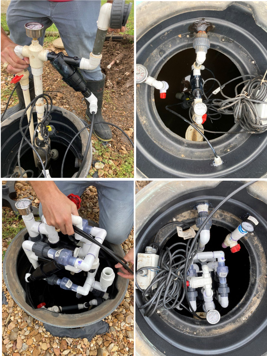
Figure 21. Installation of filters and pressure sensors on April 21-24, 2023: simple Clearstream filter, dosing to open wetland (TOP); and Clearstream Aztec Dual Spin Filter, dosing to greenhouse wetland (BOTTOM)
