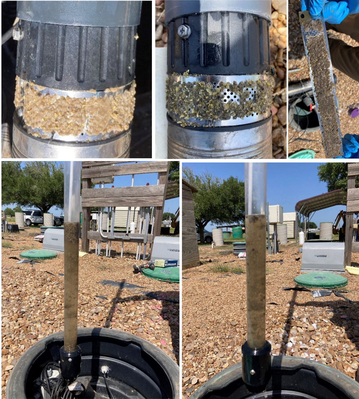
Figure 27. Pump filters clogged probably due to the combination of chicken feed and toilet paper. Chicken feed was not used anymore after the first applications: Pump filter clogged on July 14 and 17, 2023 (TOP); sludge judge test from Sc pump tank (BOTTOM LEFT) and from Sc.A/D pump tank (BOTTOM RIGHT), on July 19, 2023.
