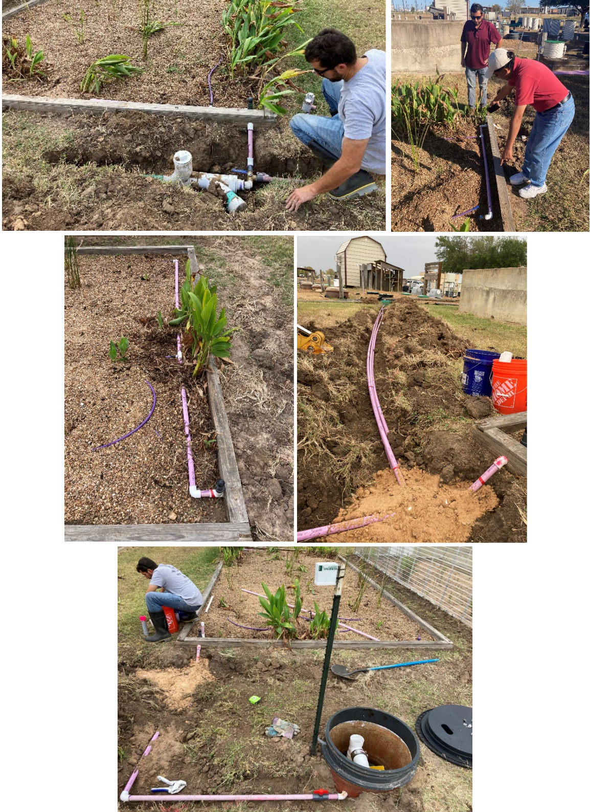
Figure 19. Connections of drip tubing in the open wetland. A manual valve can be operated to direct the flow through the original connection or the newly installed drip tubing (top left).
