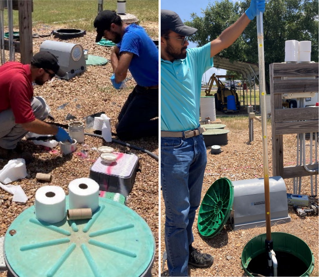
Figure 28. After initial pump filters' clogging, toilet paper started to be added in the clean outs between the trash and the aeration tanks (LEFT, July 28, 2023). Later, sludge was collected from the aeration tank instead of the MBR system (RIGHT, September 15, 2023).
