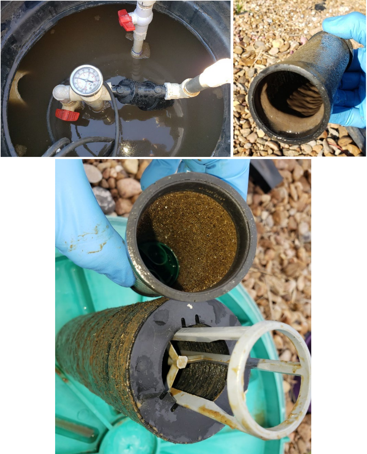
Figure 30. Pump tank high water and clogged filters a few days after capping the back filter flow: pump tank and simple screen on August 28, 2023 (TOP); simple screen and disc on October 10, 2023 (BOTTOM).
