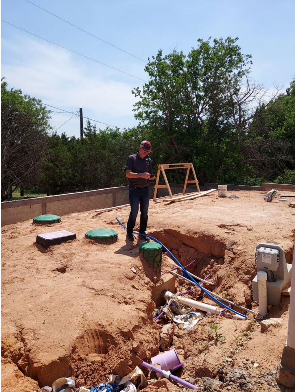
Figure 14. New Installation not in use yet (Site # 1-6).
