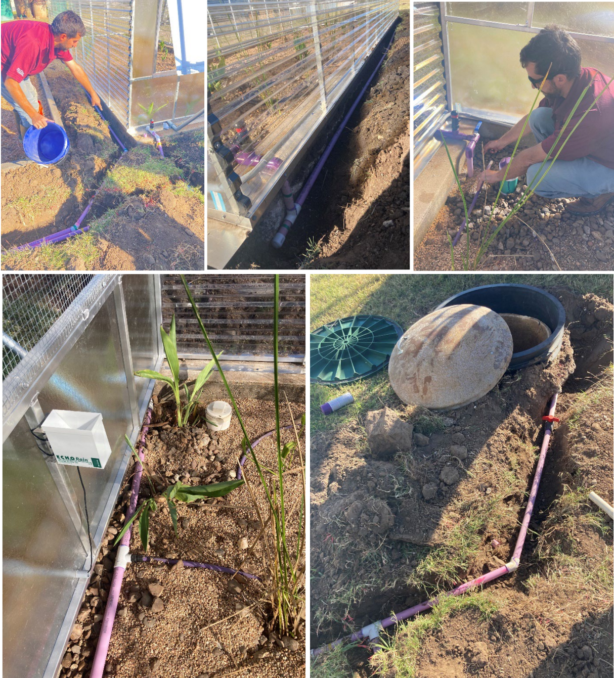
Figure 20. Connections to drip tubing in the wetland covered by greenhouse.
