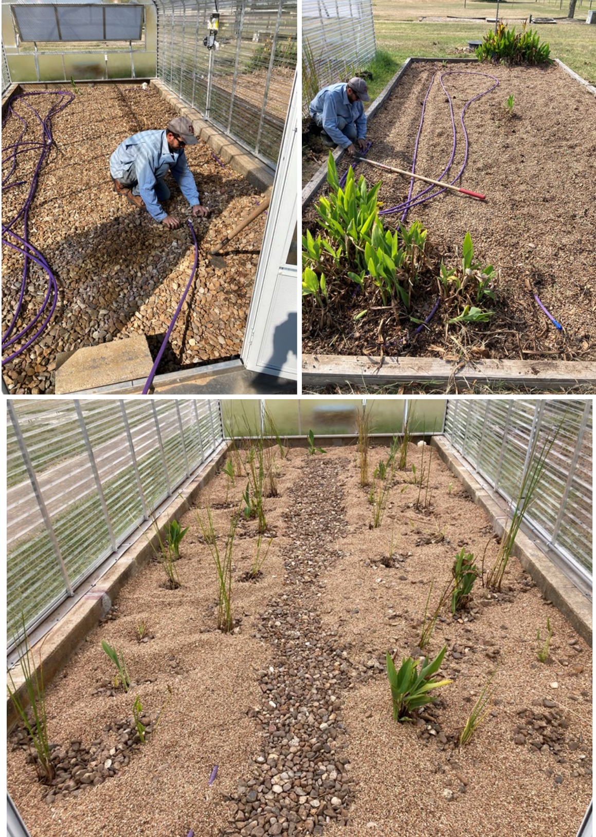
Figure 17. Installation of drip tubing on both the wetland cells (open and covered by greenhouse) on October 24, 2022.
