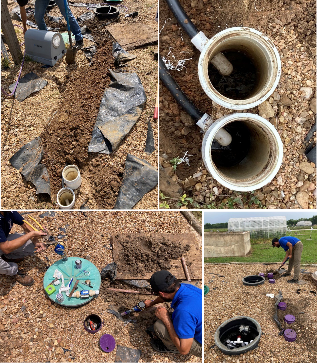
Figure 22. Installation of filter back flush lines (TOP, April 21-24, 2023) and flow meters out of the pump tank (BOTTOM, May 8-9, 2023)
