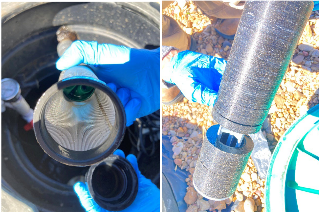
Figure 31. Once the back flush lines were reinstalled, filters looked clean again (October 17, 2023).
