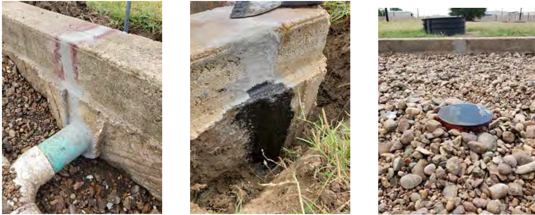
Photo 3: A few pictures of the repair work done to the concrete wall of the wetland cell.
