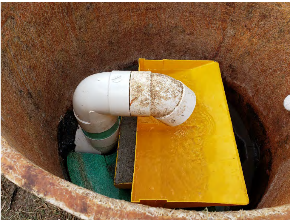
Dipper with the concrete weight installed in the wetland effluent collection tank. (Video clip is also available to see how the flow will be measured).
