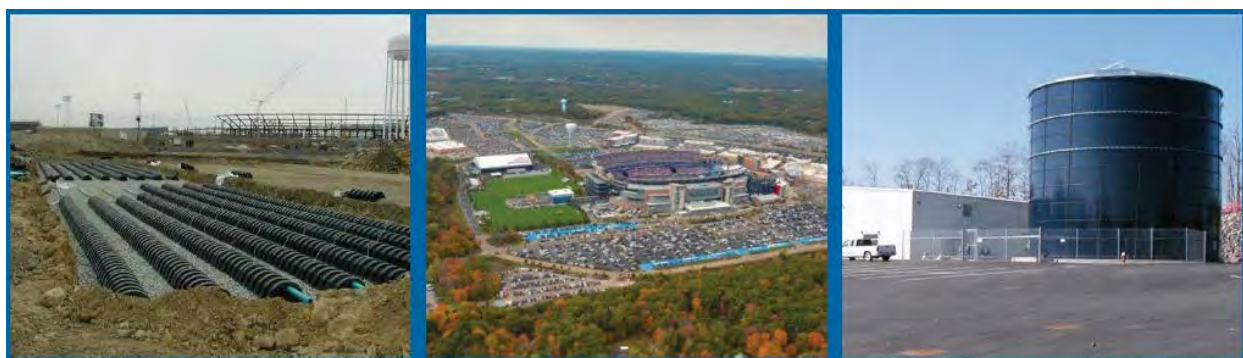
Figure 6: Installation of a chamber system under the parking lot (L), Stadium (M), and reuse water tank to meet the demand of toilet flushing. Photos are shared by Infiltrator.
