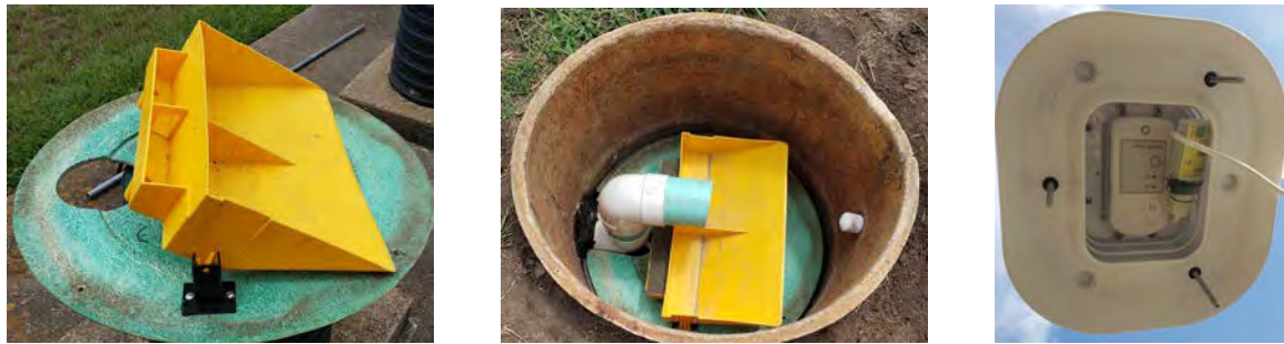
Photo 7: From Left to Right, Tipping bucket, installed at the effluent end, and Hobo data logger. NOTE: Contact Ryan to get details on how he designed and built this system!
