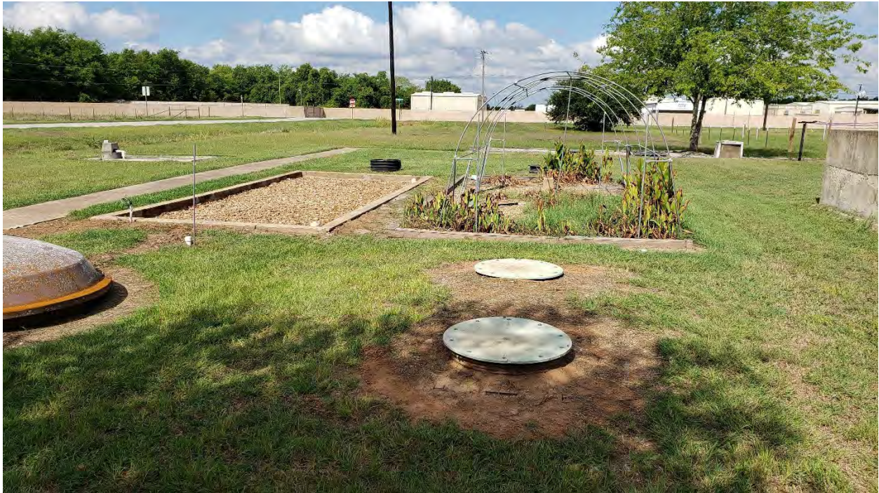
Before - Wetland cell on the left (with concrete sidewalls) ready for Greenhouse installation
