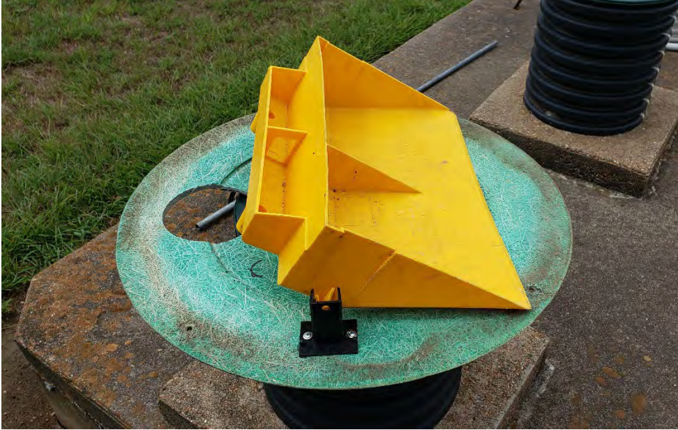
Dipper set on a riser lid, ready for installation in the wetland effluent collection tank.
