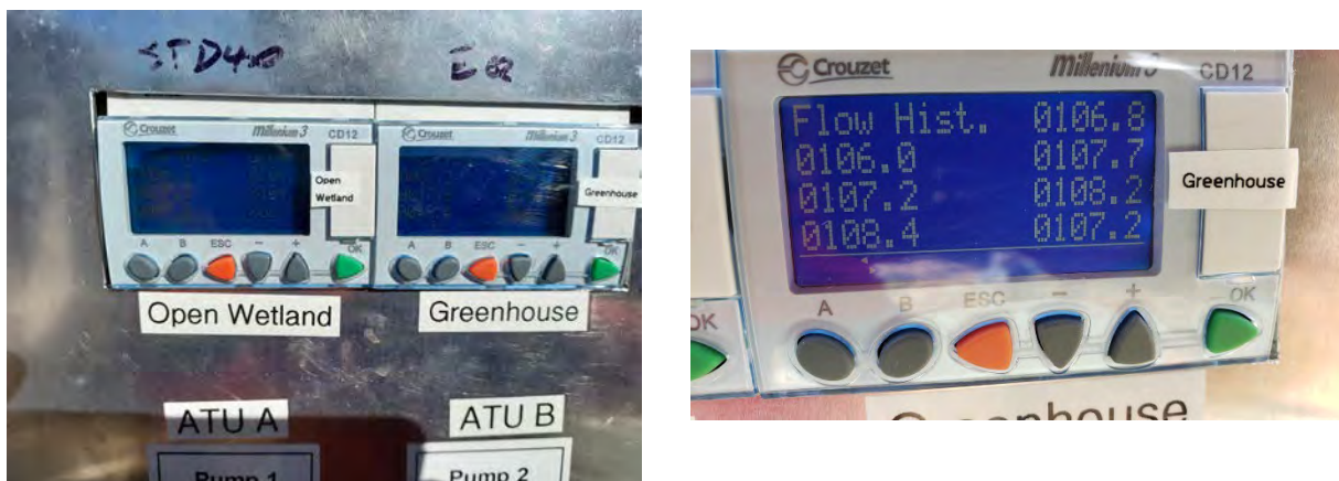
Photo 8: Digital flow recorders for influent (L), and example of the flow data for one week (R).
