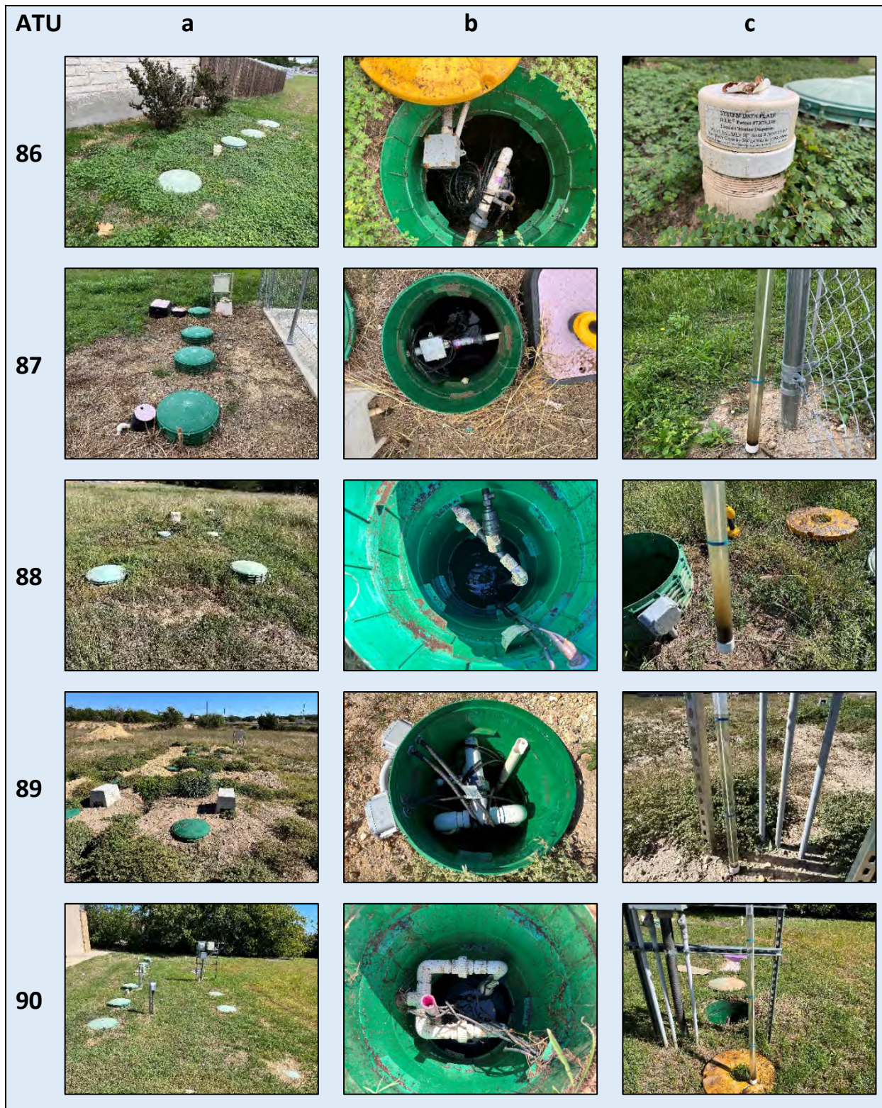
Plate 18. Photographs of ATU systems 86 through 90. Designations a, b, and c generally show a) overall system, b) pump tank, chlorinator, or lid condition or other anomaly, and c) sludge condition (if available).
