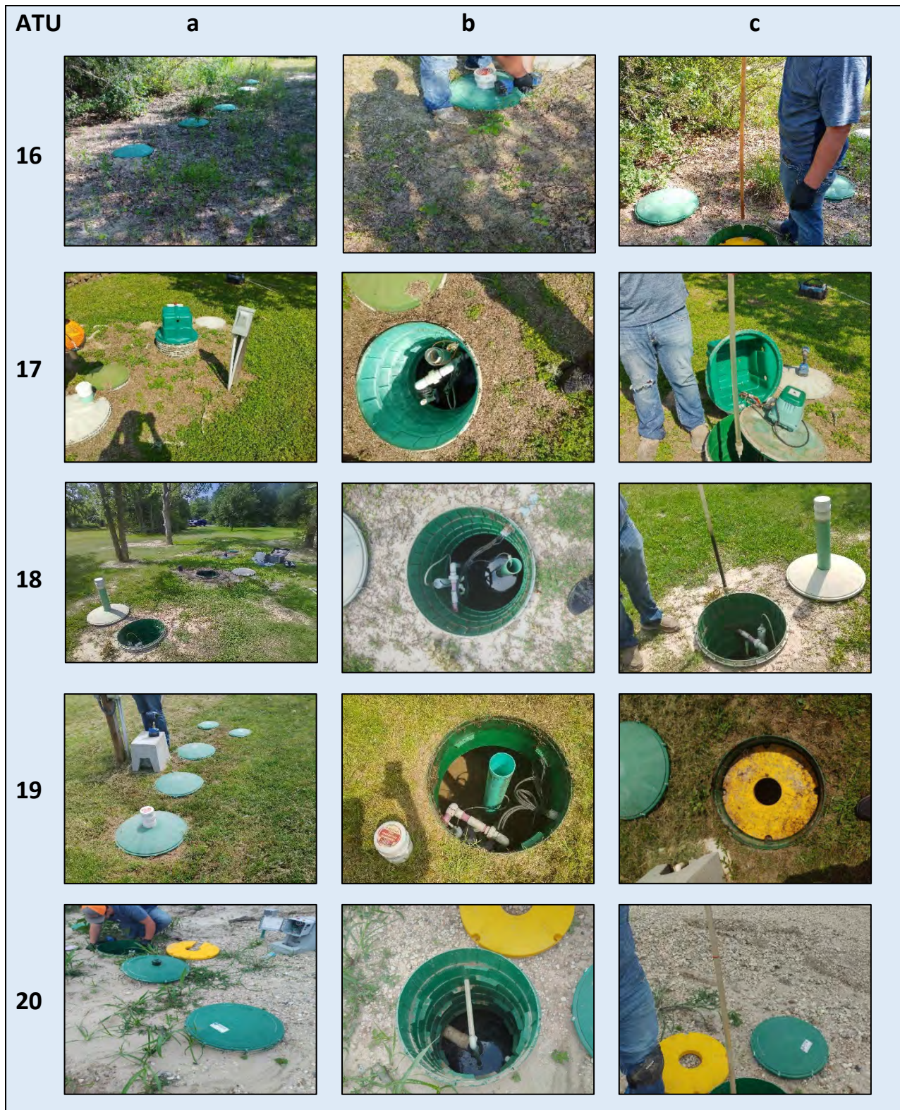
Plate 4 – Photographs of ATU systems 16 through 20. Designations a, b, and c generally show a) overall system, b) pump tank, chlorinator, or lid condition or other anomaly, and c) sludge condition (if available).
