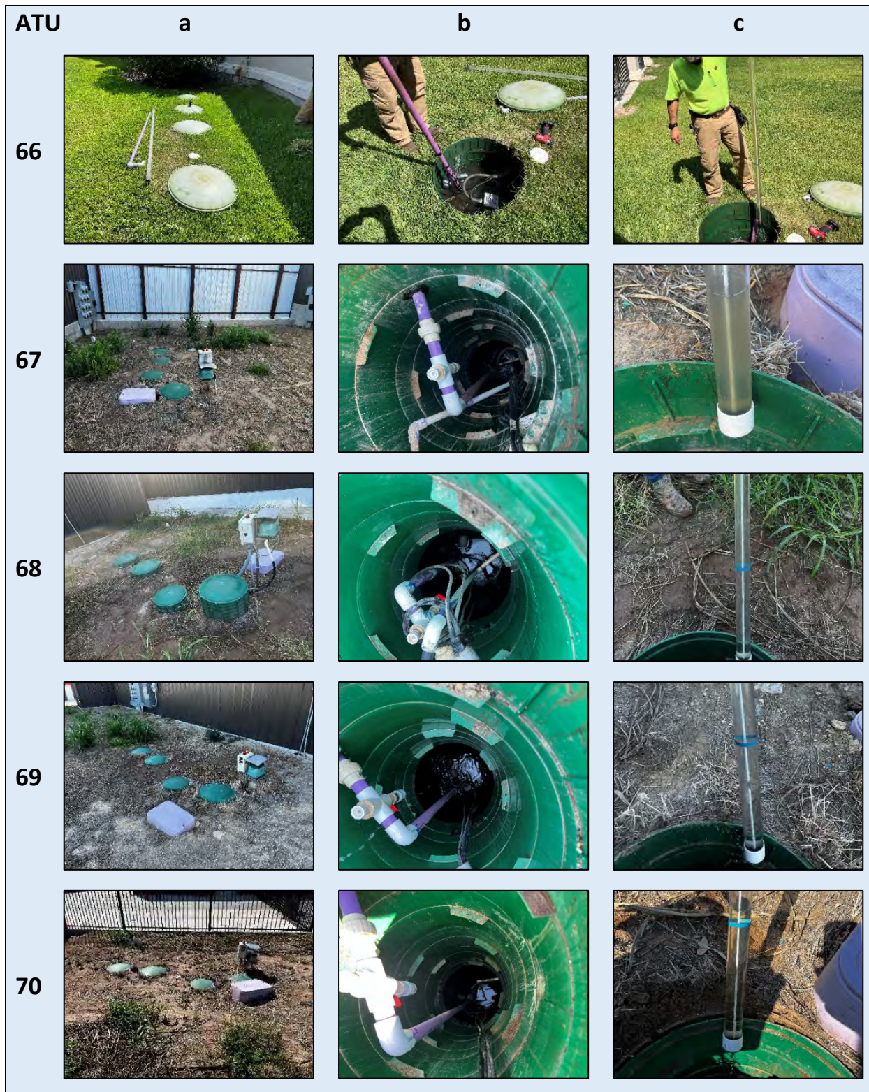
Plate 14. Photographs of ATU systems 66 through 70. Designations a, b, and c generally show a) overall system, b) pump tank, chlorinator, or lid condition or other anomaly, and c) sludge condition (if available).
