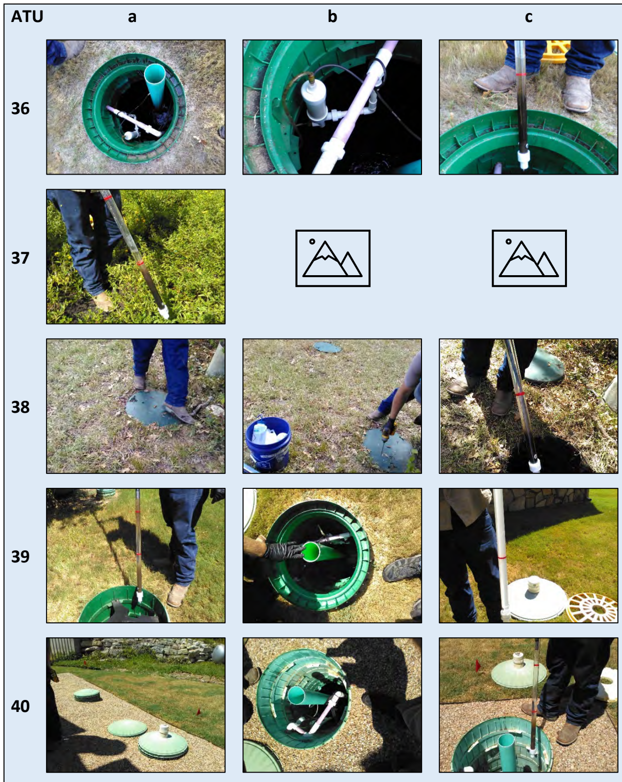
Plate 8. Photographs of ATU systems 36 through 40. Designations a, b, and c generally show a) overall system, b) pump tank, chlorinator, or lid condition or other anomaly, and c) sludge condition (if available).
