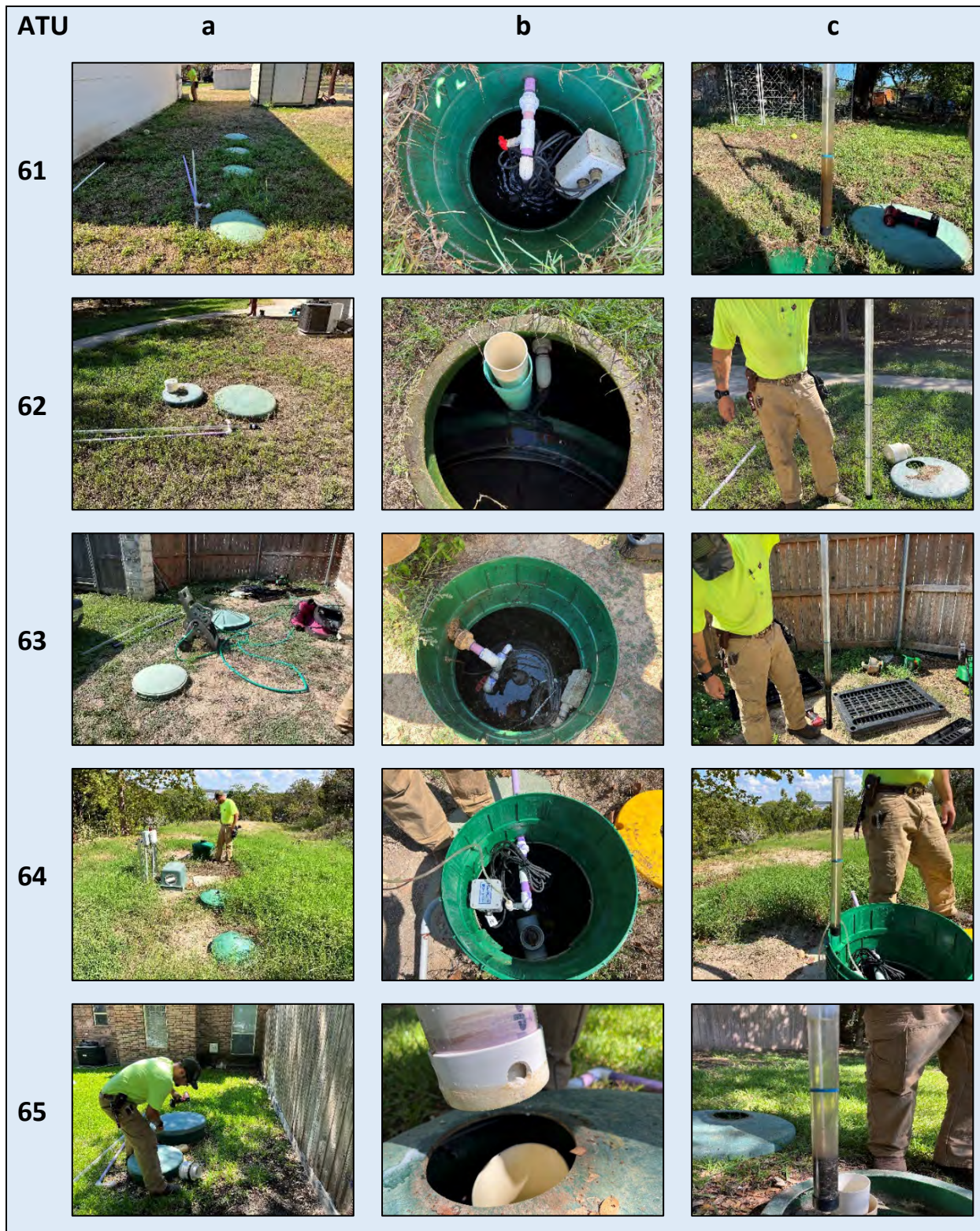
Plate 13. Photographs of ATU systems 61 through 65. Designations a, b, and c generally show a) overall system, b) pump tank, chlorinator, or lid condition or other anomaly, and c) sludge condition (if available).
