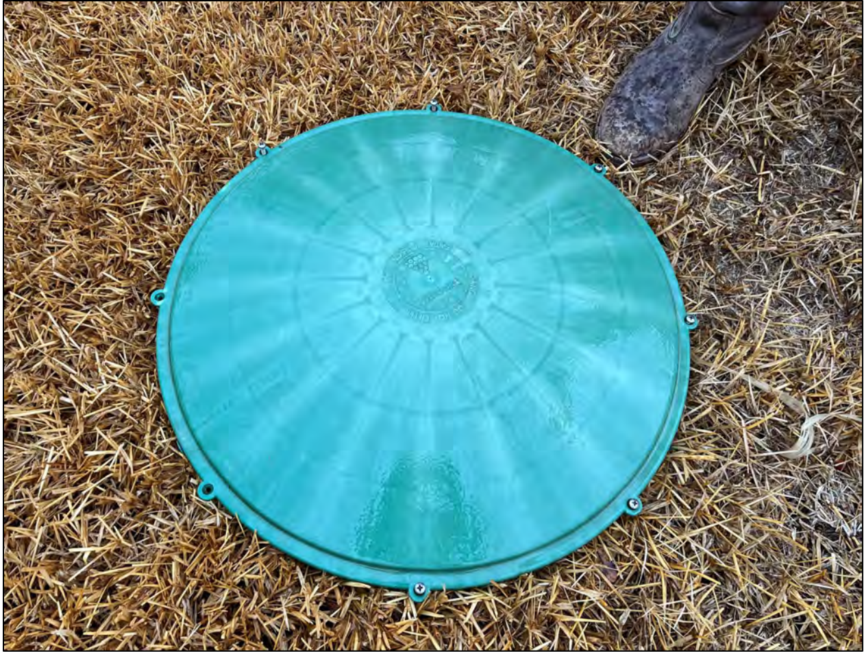
Figure 3 - ATU pump tank riser lid missing two screws at ~8 and 9 o'clock positions.
