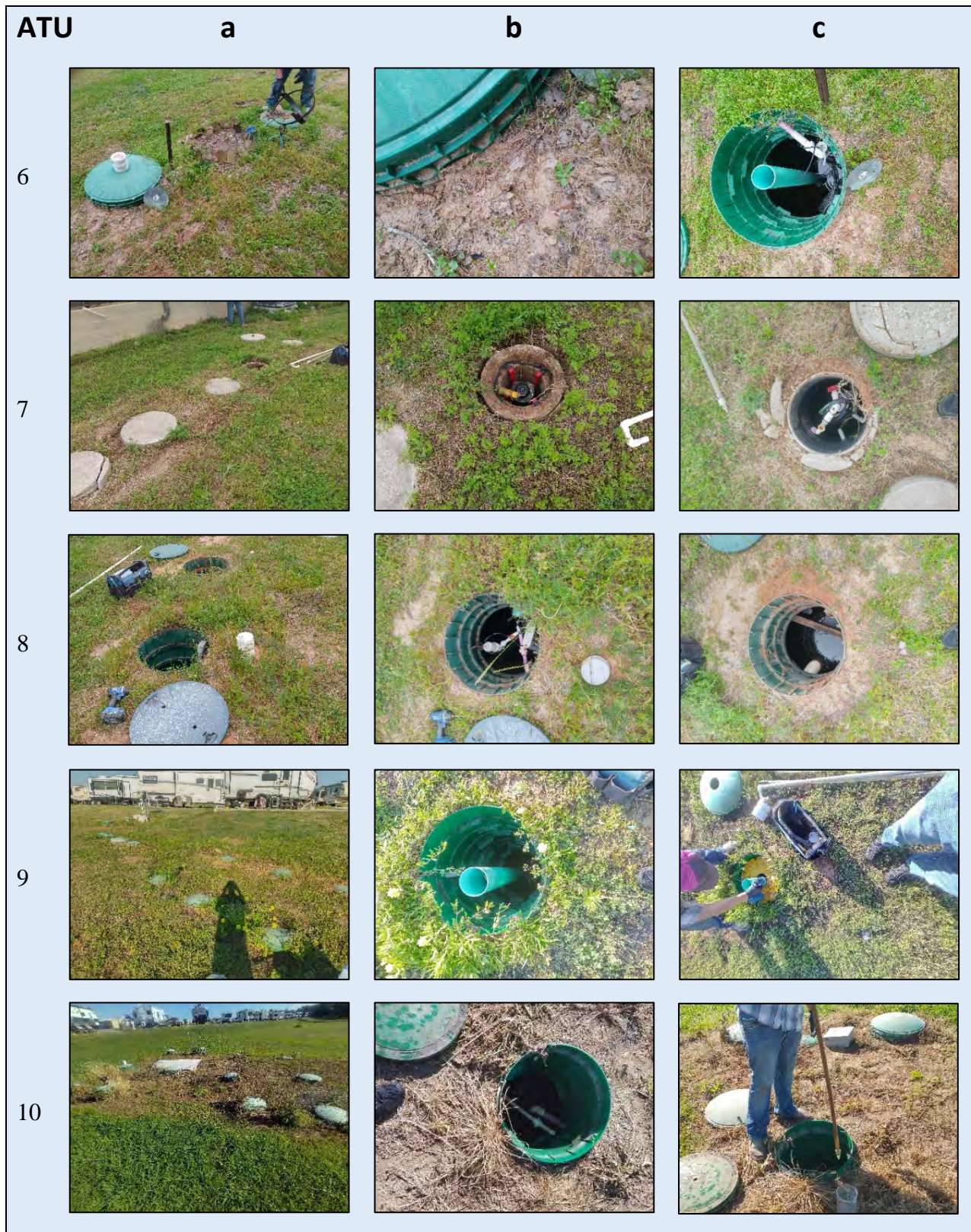
Plate 2 – Photographs of ATU systems 6-10. Designations a, b, and c generally show a) overall system, b) pump tank, chlorinator, or lid condition or other anomaly, and c) sludge condition (if available).
