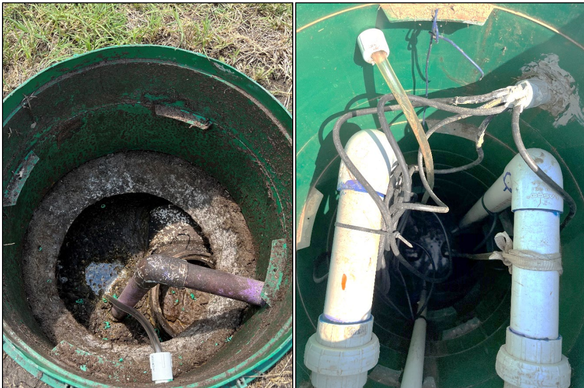
Figure 4. Vinyl sampler intake lines installed in trash tank (left) and pump tank (right).
