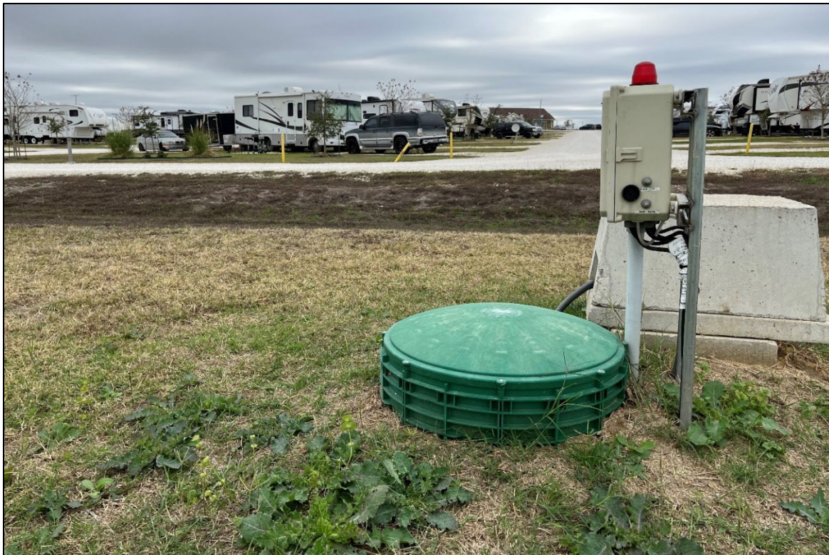
Figure 1. Texas RV park serviced by an On-Site Sewage Facility.
