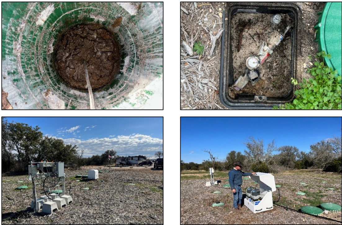
Figure 12. RV-6 Clockwise from top left; trash tank inflow line, water meter, ATU pumps, ISCO samplers.
