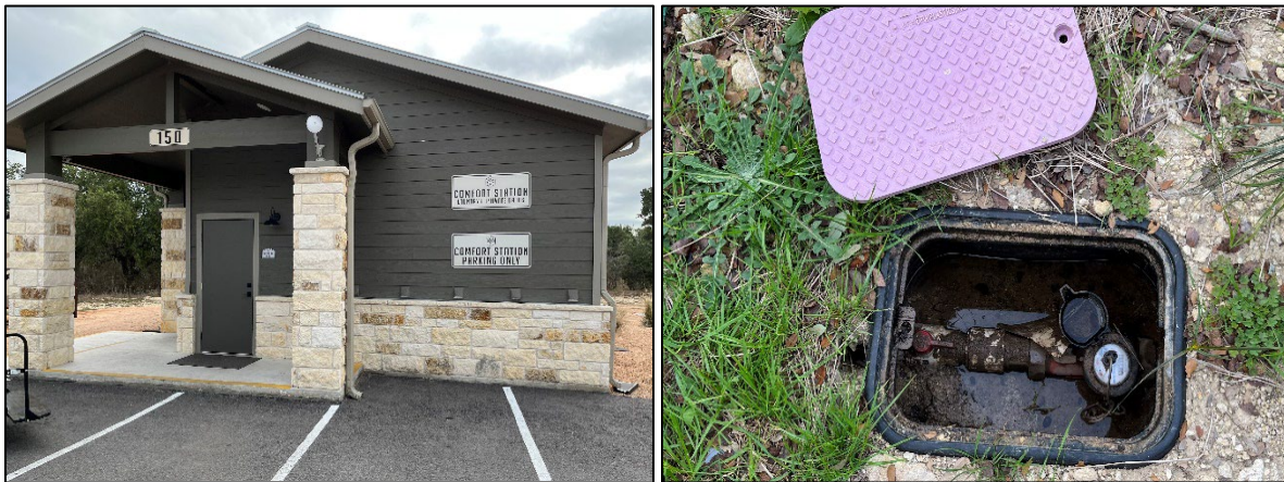
Figure 13. RV-7 Bathhouse and mechanical water meter with failed register.
