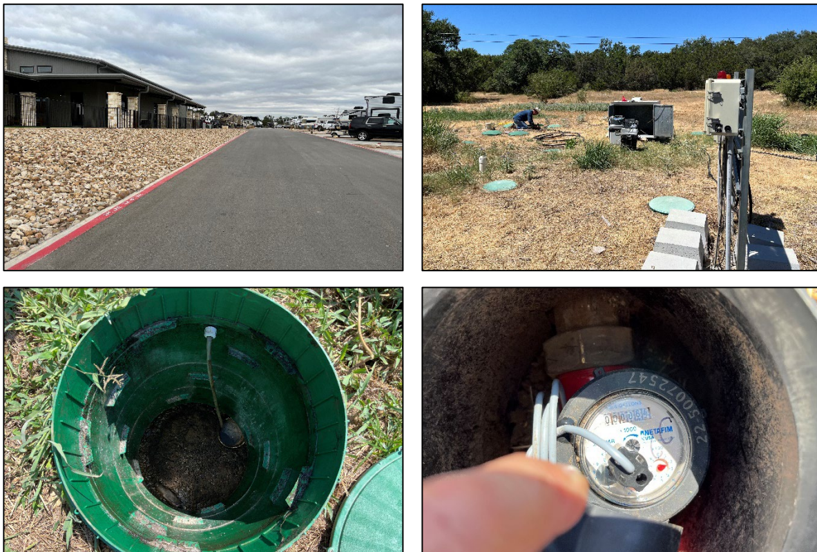
Figure 16. RV-10 clockwise from top left; clubhouse, ATU system, mechanical flow meter, and influent intake.
