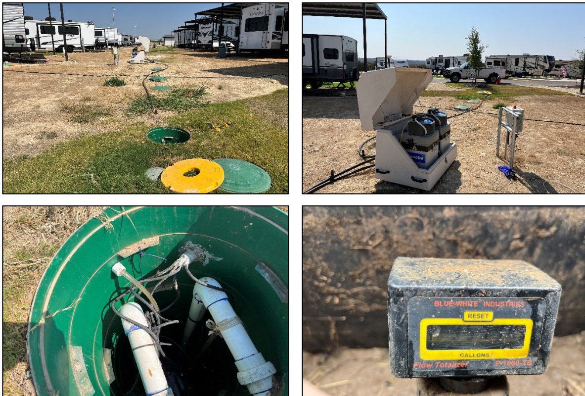
Figure 18. RV-12 clockwise from top left; overview, samplers, flow meter, and pump tank.
